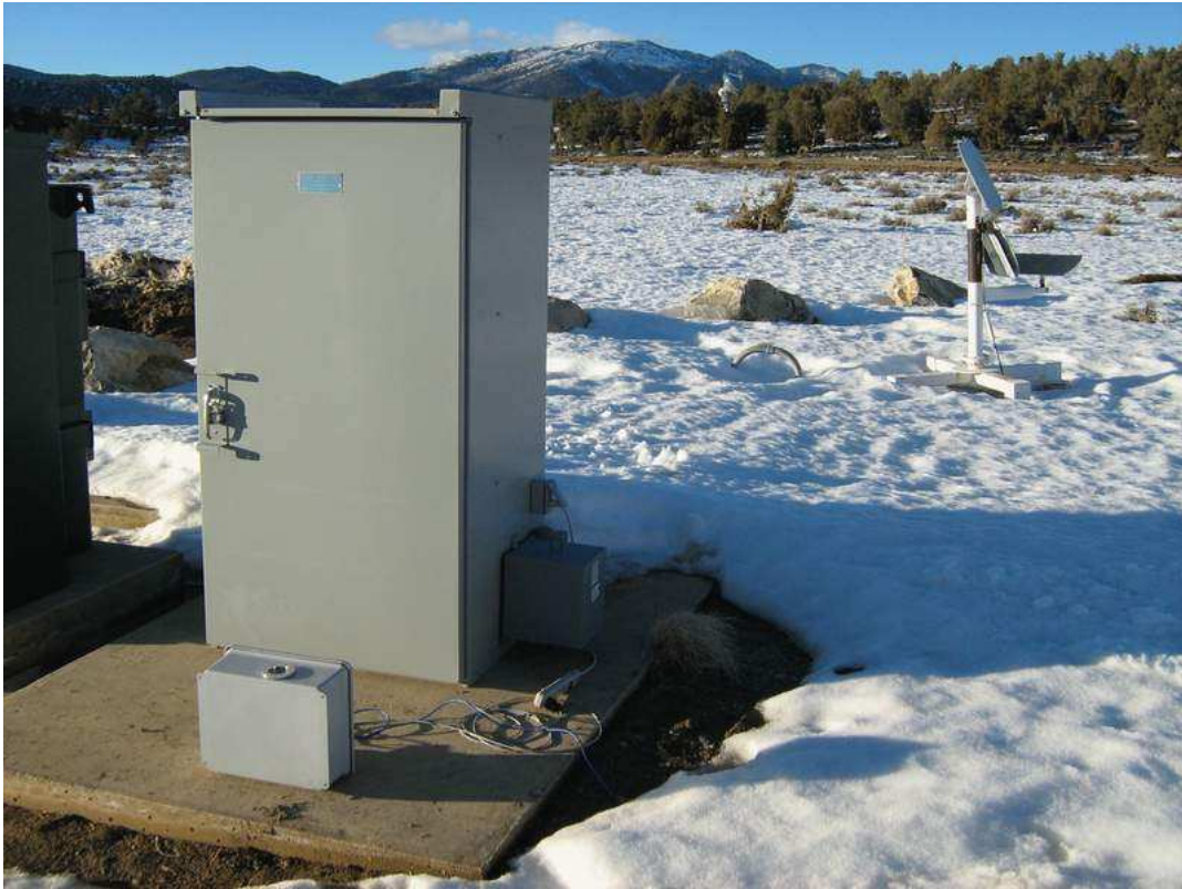
Figure 6.27 A WVR was set up near a phase monitor dish.
